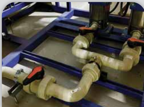
Polypropylene Type 25 ball valves and butt fusion piping in a DI water system in the medical industry
