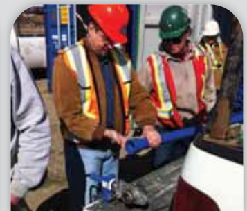
Blue PE piping for an underground compressed air system in a railway yard
