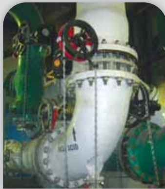
16" Polypropylene butterfly valves with chainwheel operators on a weak acid system in a sulphuric acid plant
