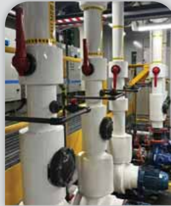
PVC ball, butterfly and swing check valves at a aquatic research centre saltwater filtration system
