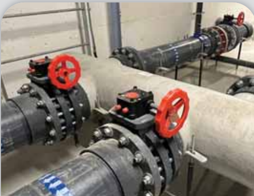
14" Polypropylene butterfly valves on a municipal swimming pool filtration system
