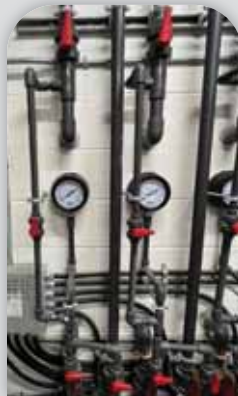
PVC ball valves on a pool sodium hypochlorite chemical injection system
