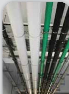
Pre-Insulated PP-RCT pipe and PP-RCT piping installed in a chilled water system
