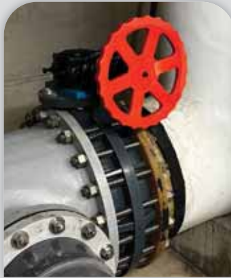
24" PP butterfly valve installed in an aquarium saltwater filtration system
