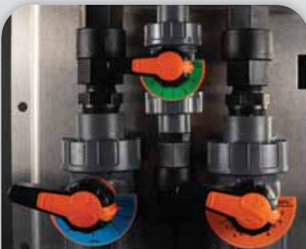
SM Series PVC metering ball valves installed on a pressure washing manifold system
