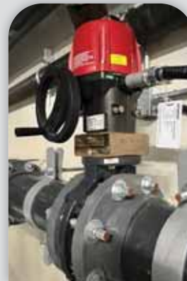
Actuated butterfly valves on a municipal swimming pool filtration system
