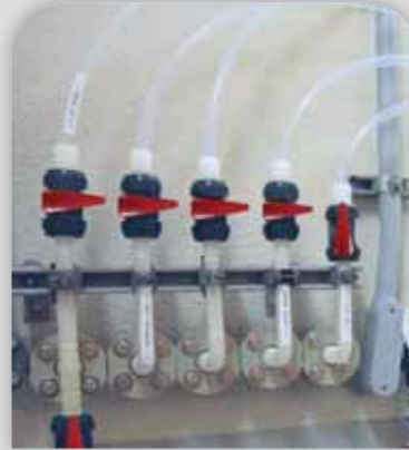
ChemFlare™ System (valves, fittings, tubing) for sodium hypochlorite in a water treatment plant
