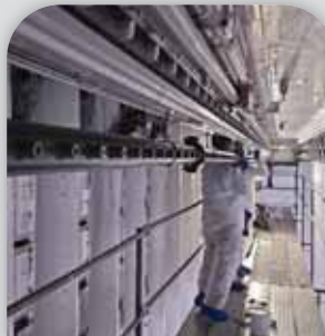
PVC manifolds with spigot ends in a vertical hydroponic operation
