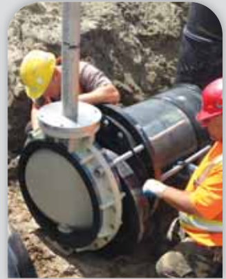
18" PP butterfly valves with stainless steel stem extensions for a landfill methane collection system
