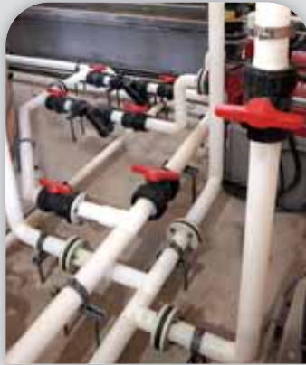
ECTFE (Halar®) pipe and fittings for sodium hypochlorite piping system in a sewage treatment plant
